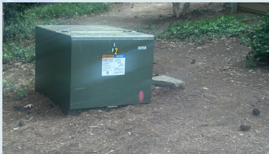
Single Phase Pad Mounted Transformer in Large Apartment Complex
